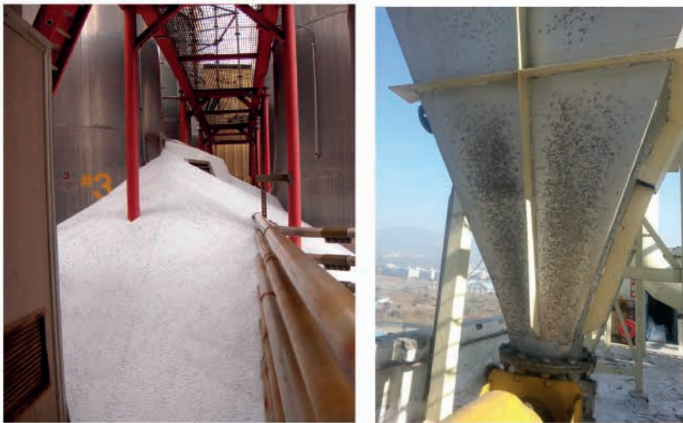
Flooding (left) and erratic flow/stoppages, as evidenced from hammer rash (right), are just two of the problems routinely associated with sub-optimal hopper design and/or operation.
